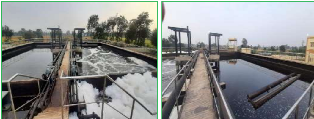
Rajnadgaon (Mohad): 6.2 MLD
